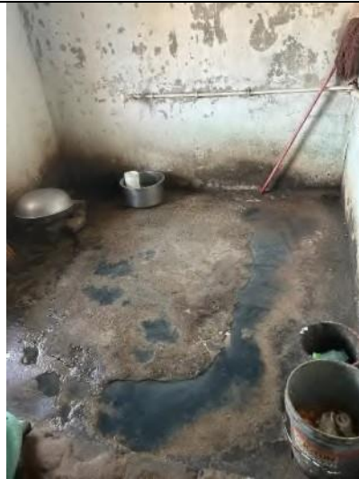
Unhygienic conditions in the utensil washing area
