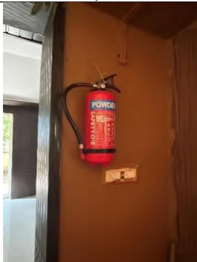
Adequate placement of fire extinguishers
