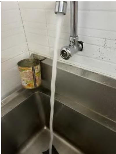
Aerated taps in kitchen washing area
