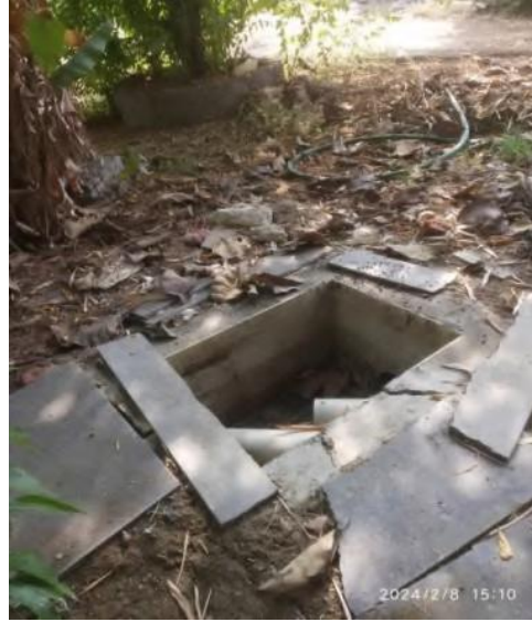
Open Septic tank
