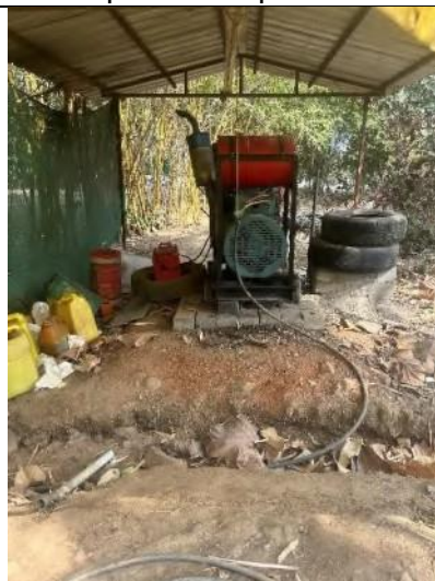
Waste dumped near th D.G set
