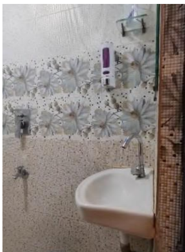
Soap dispenser in guest washrooms
