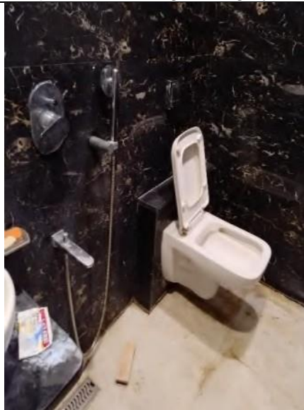
Dual flush system in all washrooms
