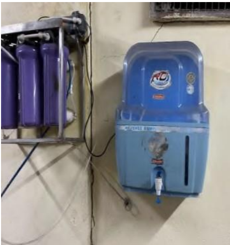
RO filter for water consumption
