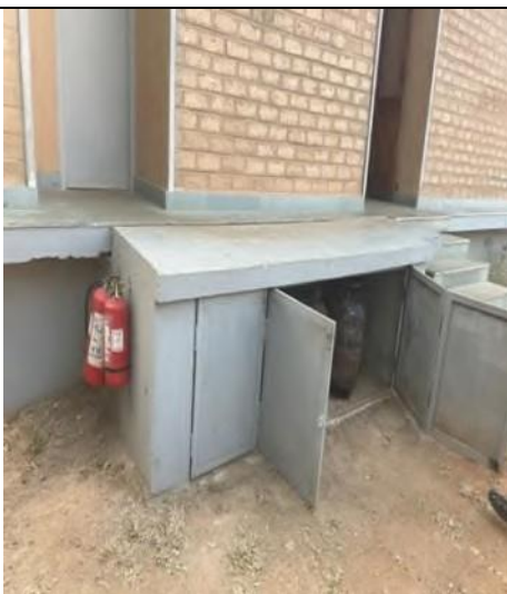
Fire Extinguishers near Cylinder Store
