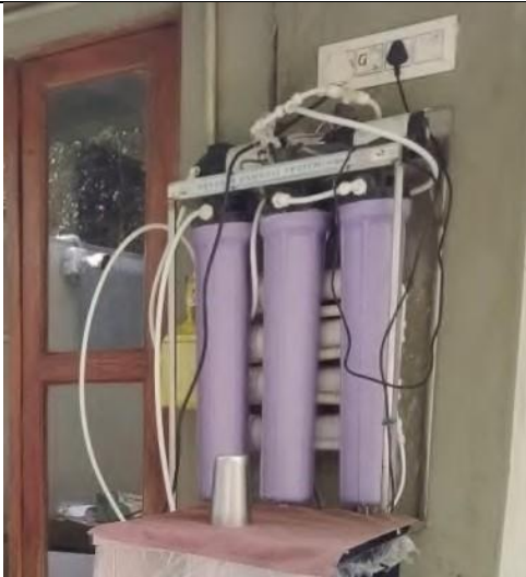
RO filtration system
