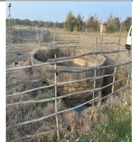
Damaged Well, requiring maintainance
