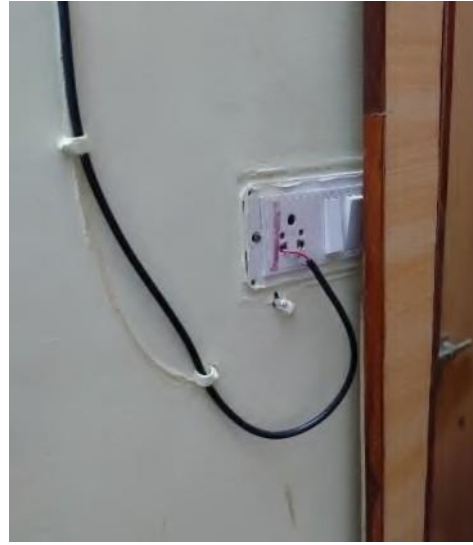
Live wires in the guest rooms
