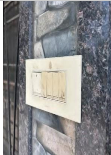
Single switch in visitor room
