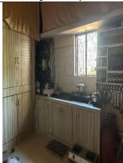
Absence of fire extinguisher in kitchen
