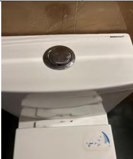
Dual flush in washrooms
