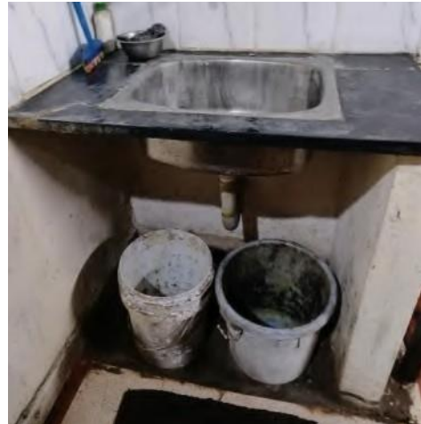
Unkept utensil washing area
