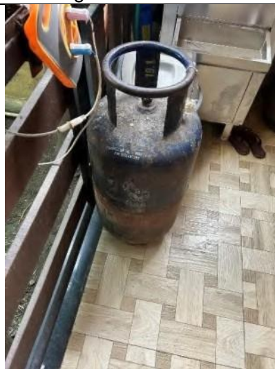
Absence of fire extinguisher near the cylinders
