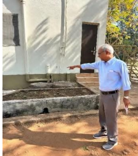
Uncovered Wastewater Channel
