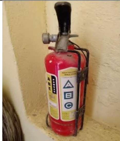
Old fire extinguisher
