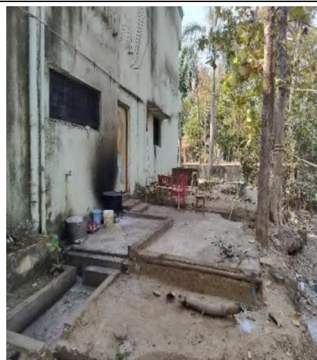
Burning of waste and unkept open areas
