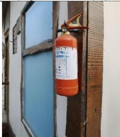
Absence of expiry date on fire extinguishers
