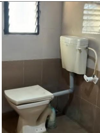
Single flush in washrooms
