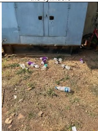
Plastic waste dumped near th D.G set
